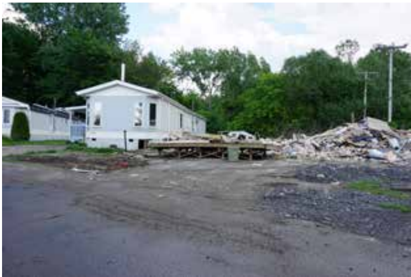
Right: The dike breached at the trailer park. Some trailer homes were heavily damaged and were demolished when the floodwater resided.
