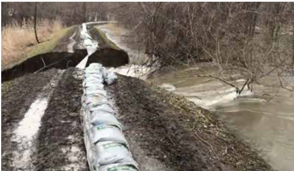
Below: The 20m wide dike breach (Pilon, 2019b).
