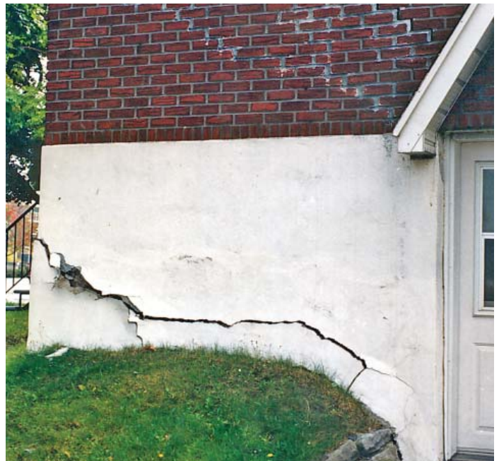
Cracks in wall likely due to shifting foundations Credit: © Ville de Montréal
