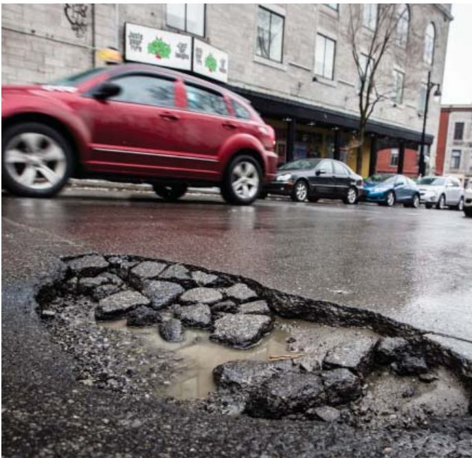
Pothole on St. Lawrence Blvd., near Sherbrooke St. (25.02.2013) Credit: © Dario Ayala, Montreal Gazette
